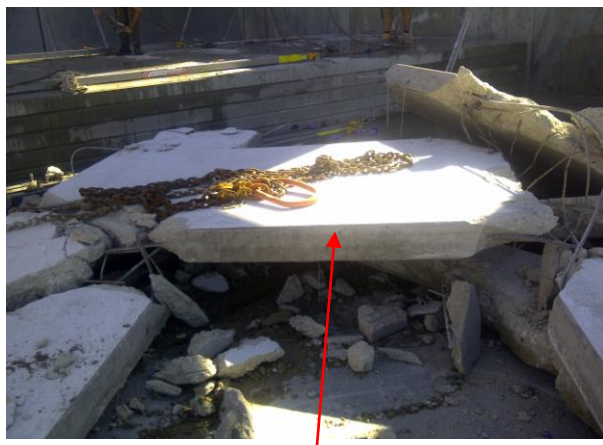
Resulting damage to panel after incident
